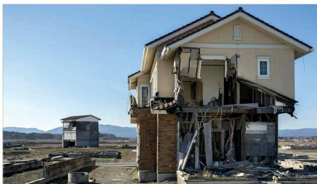
Figure 2. A destroyed house (Javier Tles) https://english.elpais.com/elpais/2016/05/02/inenglish/1462201618_695572.html
